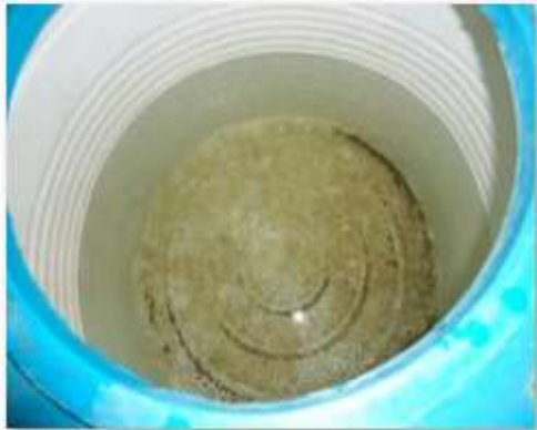
Condition of Drinking Water Storage at Moirang High School
